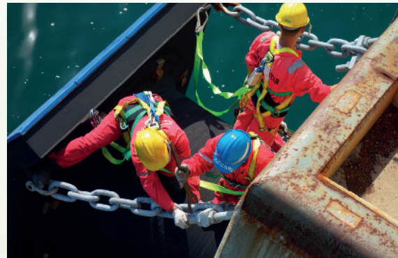
Harbor Star Maintenance Unit doing remedial repair tensioning for fender in GNPower, Mariveles
